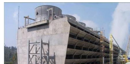
Pipe racks for oil companies, water storage and water-cooling towers for power plants.
