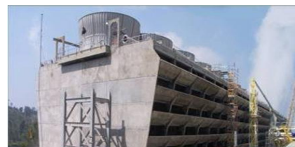
Pipe racks for oil companies, water storage and water-cooling towers for power plants.
